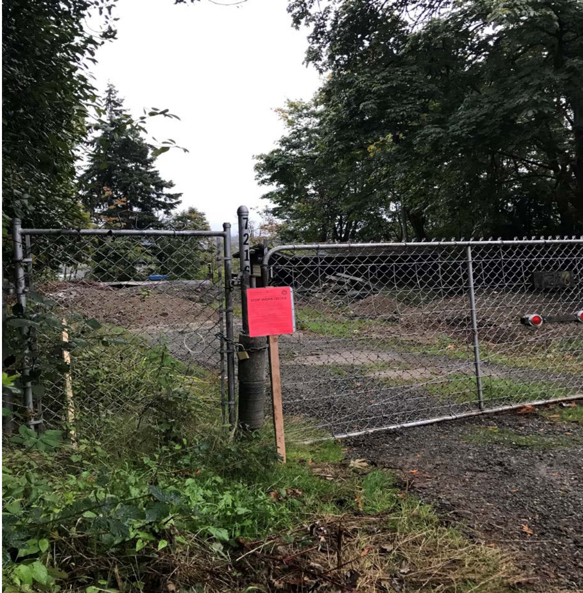
Exhibit 1-D: Second Stop Work Order Posted Photo taken 10/19/2020.
