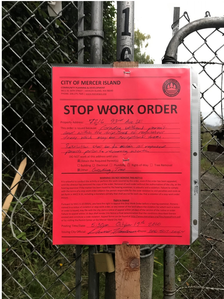
Exhibit D: Second Stop Work Order Posted Photo taken 10/19/2020.
