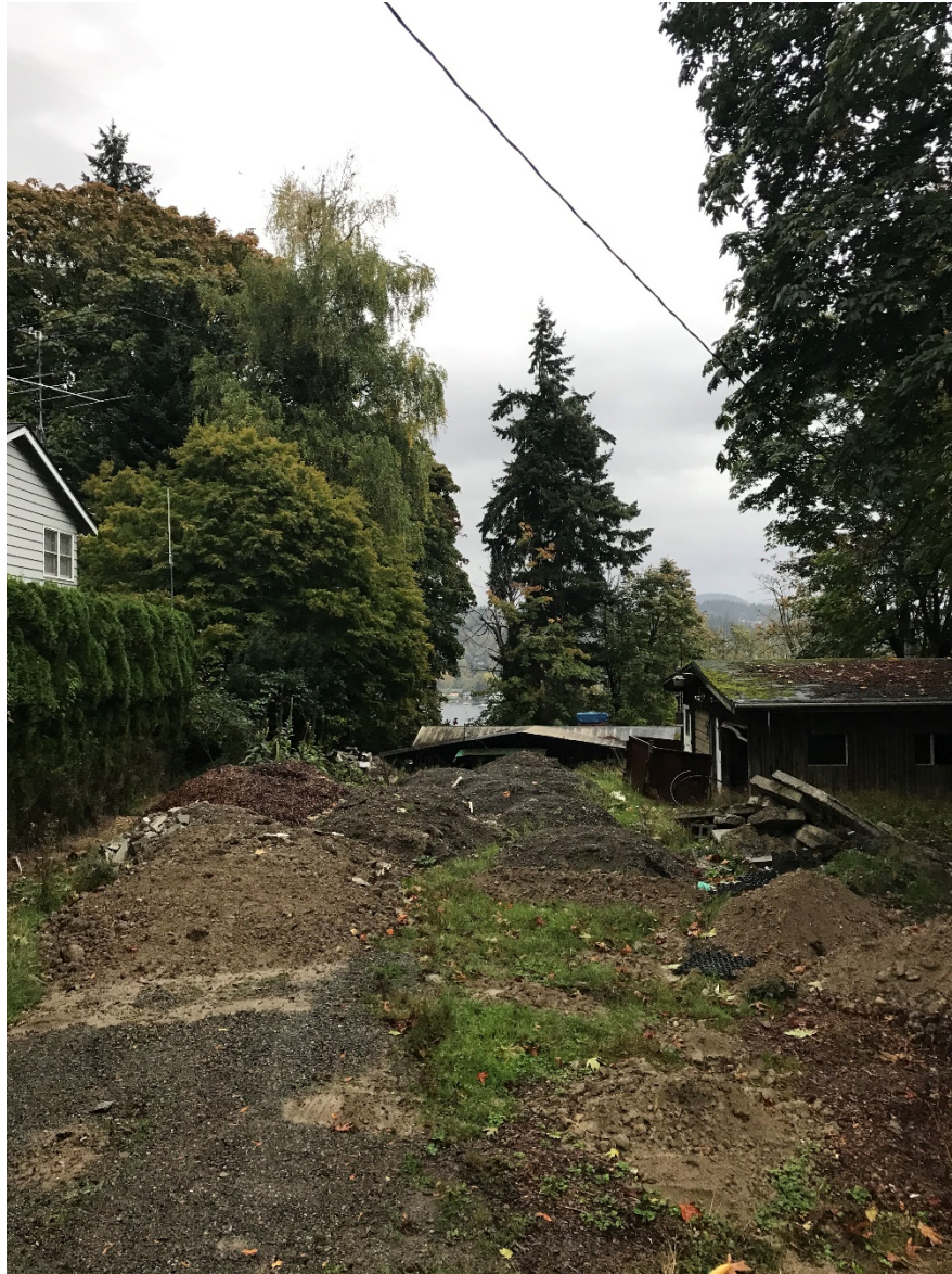
Exhibit 3-D: Second Stop Work Order Posted Photo taken 10/19/2020.
